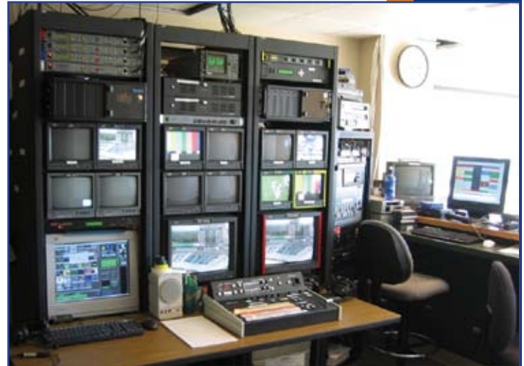
Floyd Casey Stadium Control Room
