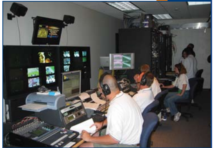
Kinnick Stadium Control Room
