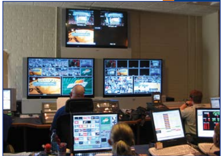
Allen Fieldhouse Digital Control Room
